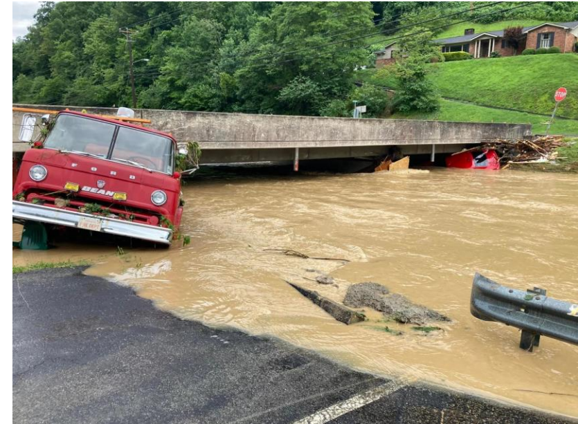
Floodwaters surround vehicles and a bridge in Hindman, Kentucky, during the July 2022 Eastern Kentucky flood. Photo by Tyler Wolfe
