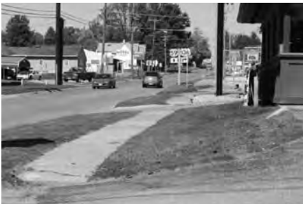
NW Missouri COG - Sidewalk Assessments, fair condition
