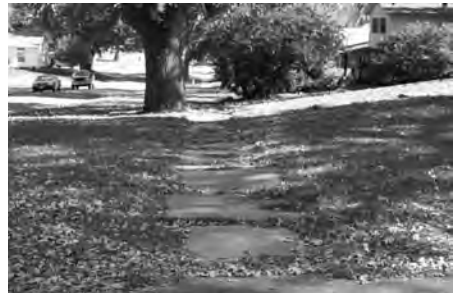
NW Missouri COG - Sidewalk Assessments, poor condition
