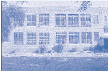
Rehabilitation of the Old West End School in North Carolina is under construction to develop 10 elderly apartments and expand Senior Center space for activities including space for a new Adult Day Care.
